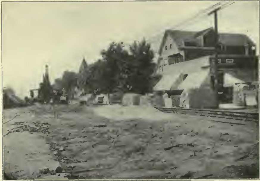
FIG. 51. STREET CONSTRUCTION, A SOURCE OF DUST. More than a million square yards of street repairs are made annually in Chicago. In this view a six-foot brick sewer is being laid, after which the street may long remain in the disturbed condition shown. During construction, dust is distributed about the neighborhood from the handling of cement, brick and sand. Photograph taken August 21, 1914.
